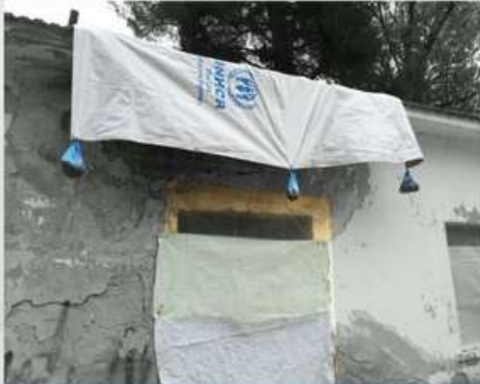
Refugees creatively try to solve broken windows and roof openings to protect themselves
